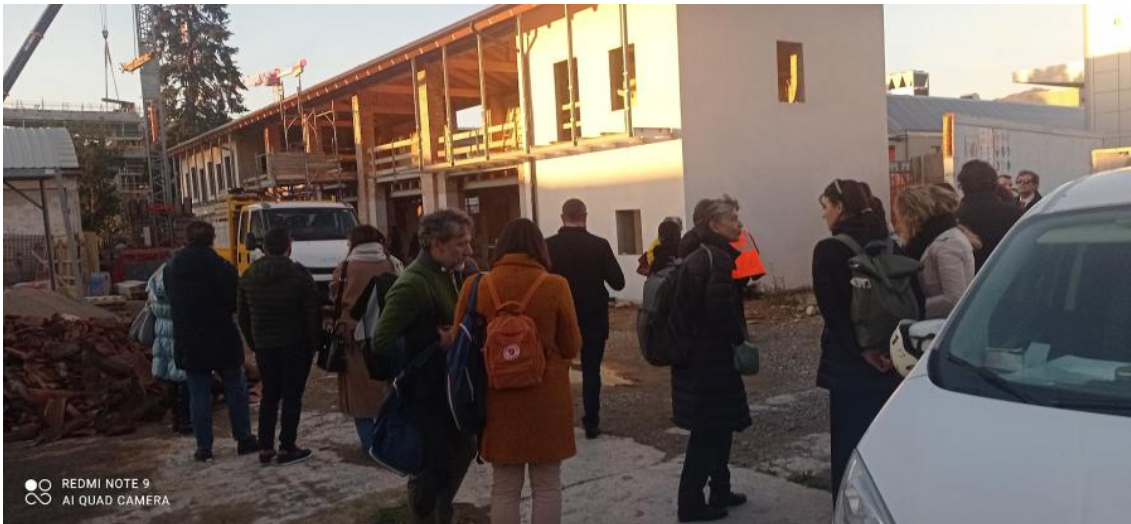
Representative of Italian municipalities visiting the building site of the Hub4Kids in Via Serassi
