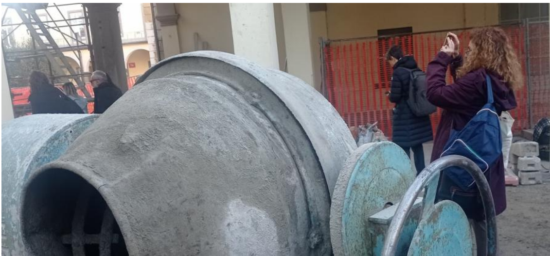
Representative of Italian municipalities visiting the building site in Borgo Palazzo, place of the co-housing experience, former hospital
